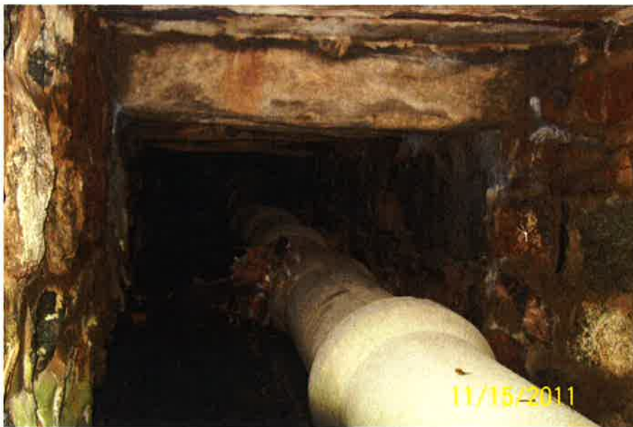
Photo No. 12– Concrete pipe extending in culvert barrel (beyond view DIP/CIP cross-through pipe below concrete pipe).
