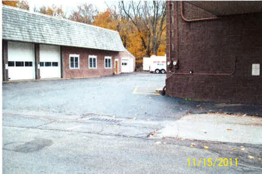
Photo No. 1 – View across the Firehouse Parking Lot looking from Main Street culvert to stone masonry channel at the stream corridor.
