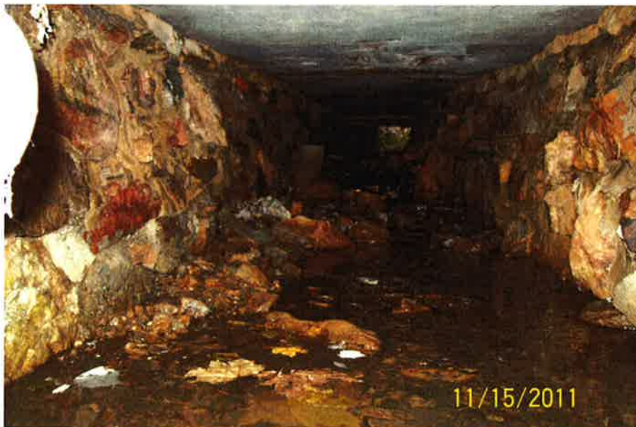
Photo No. 8– Upstream view of the first reach from inlet (similar to downstream view from inlet).
