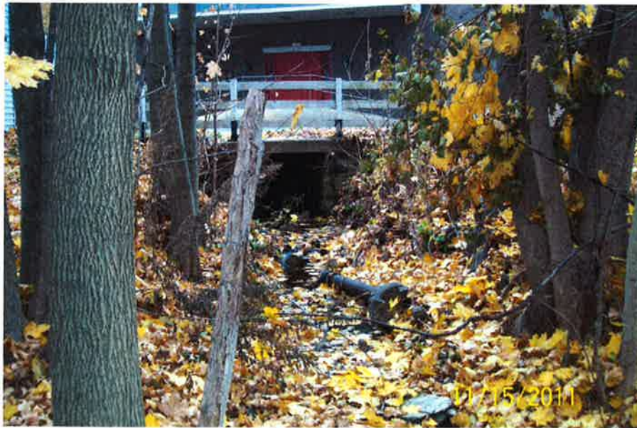
Photo No. 10– View of Main Street culvert downstream headwall and receiving channel.
