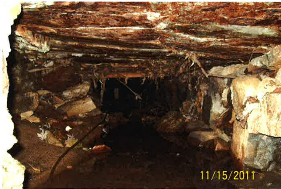
Photo No. 7– Downstream view of the first reach of the stone masonry culvert under the Firehouse Parking Lot.
