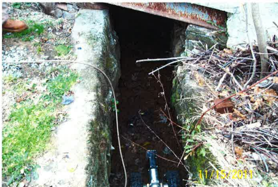
Photo No. 6– Stone masonry channel opens to a wider stone masonry culvert under the corner of the Firehouse.
