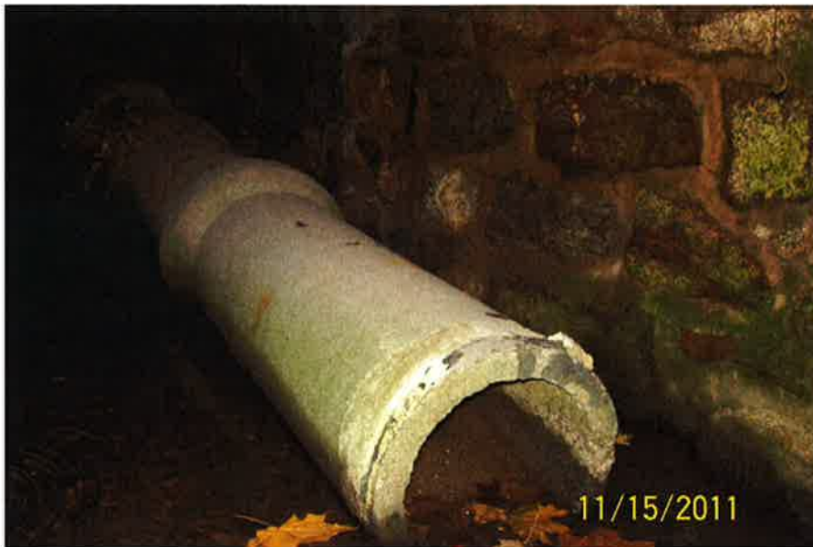
Photo No. 11– Concrete pipe in barrel of Main Street culvert at downstream end.
