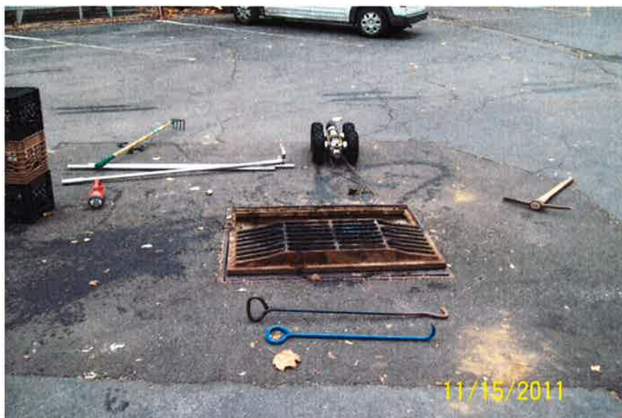
Photo No. 3 – Inlet located in the Firehouse Parking Lot served as a second access point to the system (camera unit in background).
