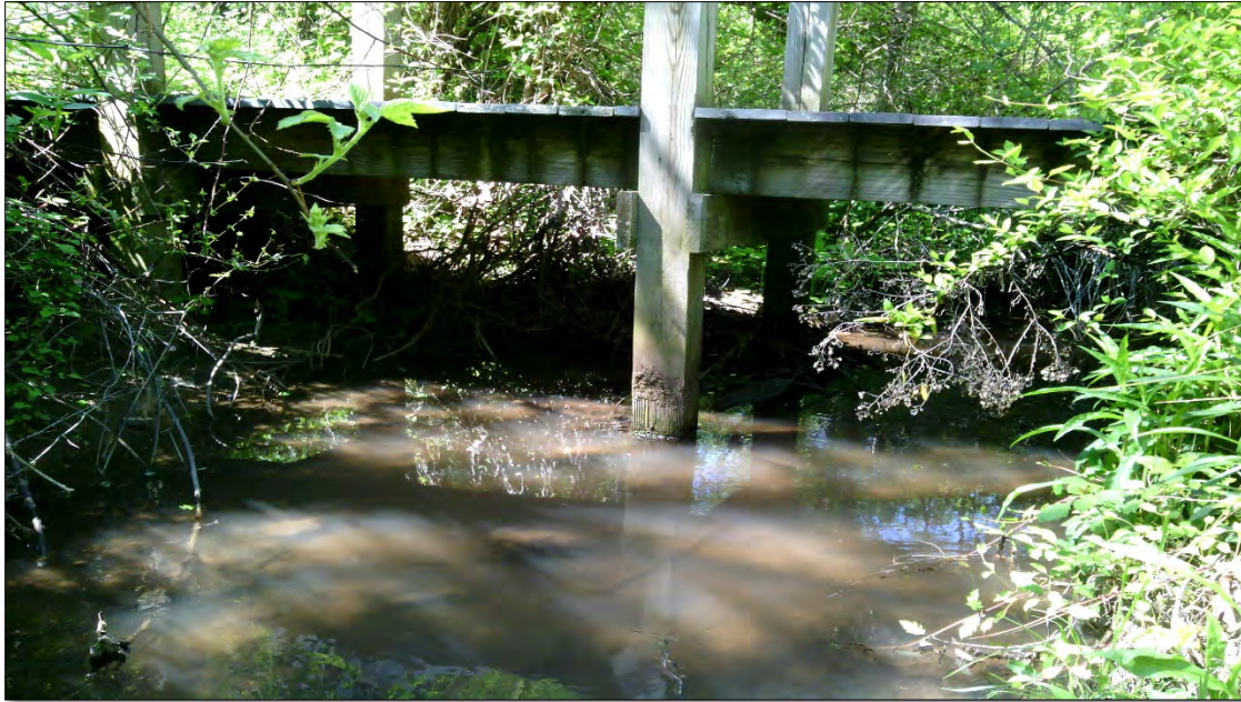
Photo 7: View north and upstream at a footbridge observed across Reach-01 connecting a mown path through open space to a shopping center.
