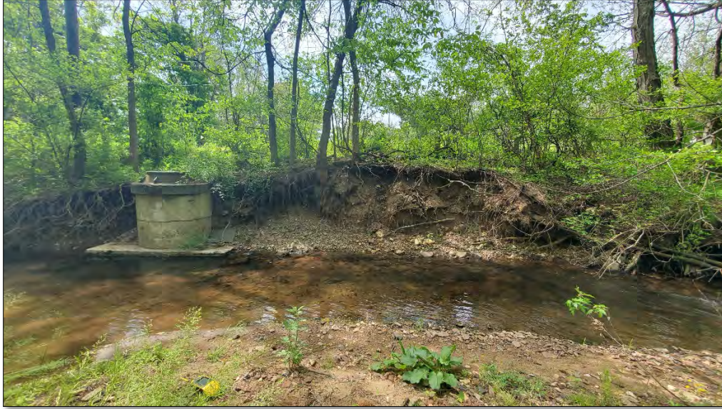
Photo 9: View south at bank erosion on right bank of Reach-02 exposing sewer manhole.
