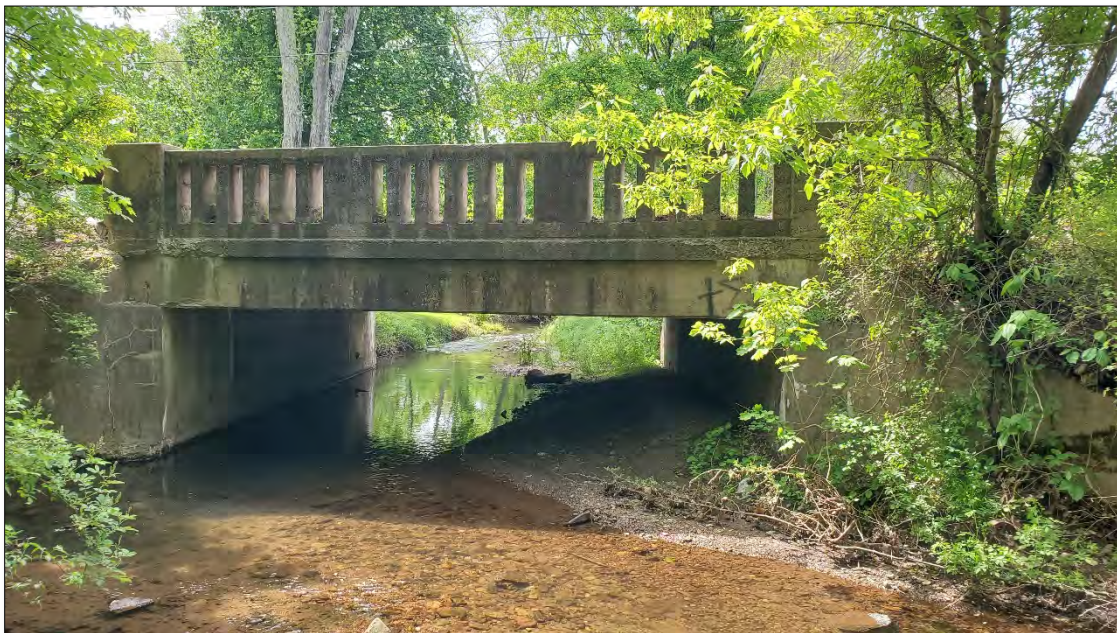
Photo 6: View south and downstream at an example of a bridge across Reach-02 at the Main Street crossing.
