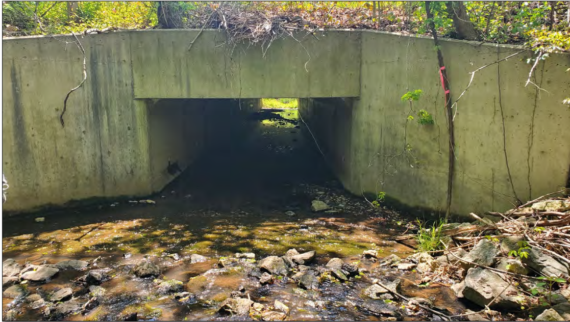
Photo 5. View south and downstream at an example of an undersized box culvert on Reach-01. Note CPOM deposited at top of culvert.
