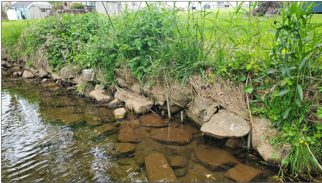
Photo 12: Bank armoring observed along the left bank of Reach-02.
